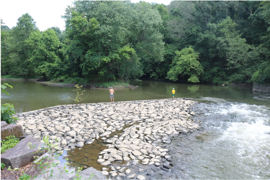
Augustine Dam 3, breached
