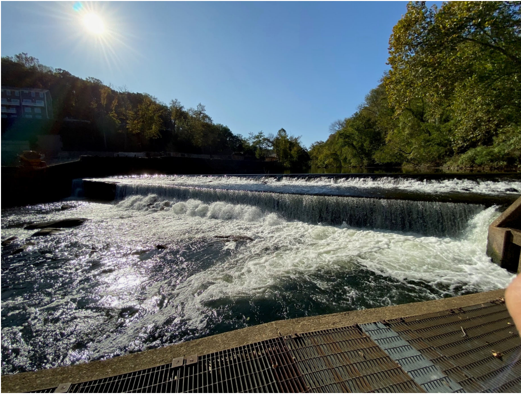
Bancroft Dam 4, damaged in center of dam
