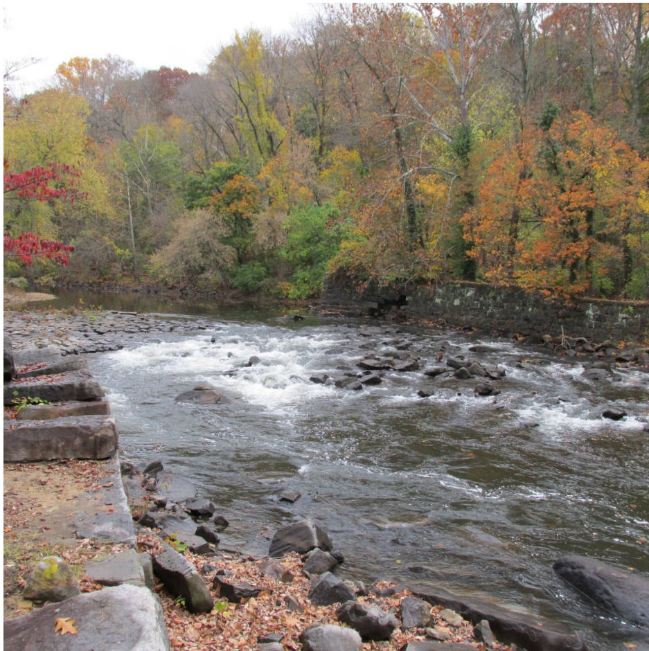
Augustine Dam 3, breached
