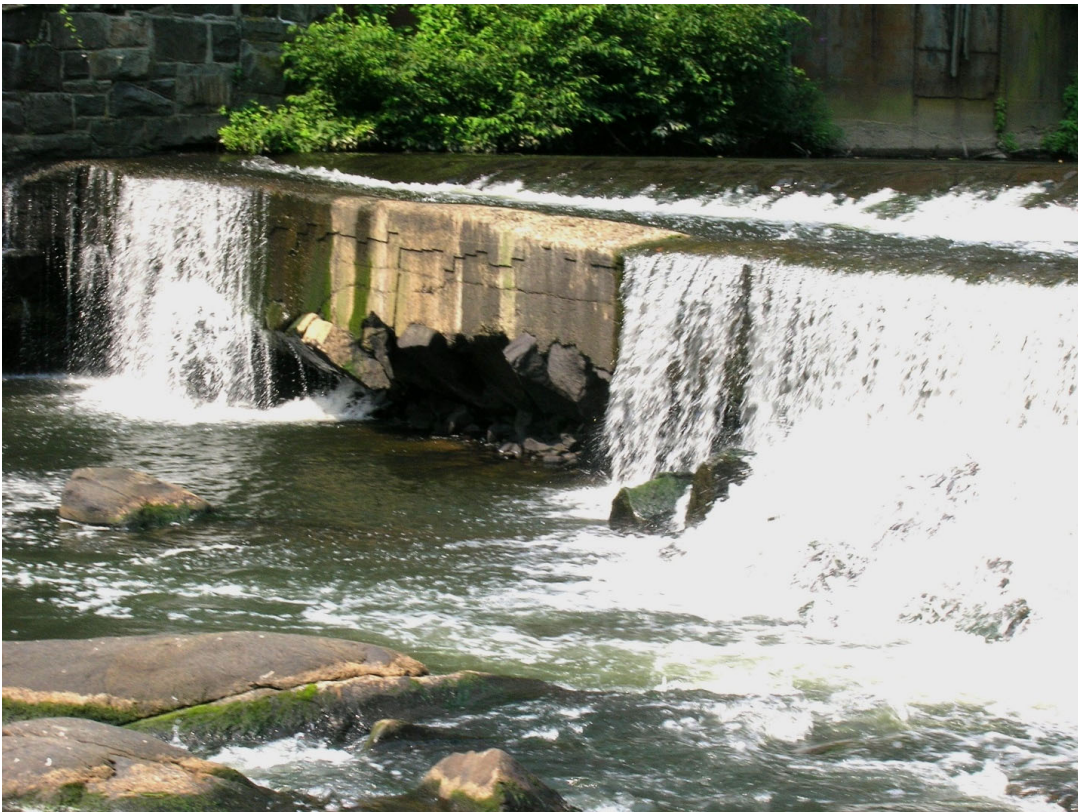
Bancroft Dam 4, damaged in center of dam
