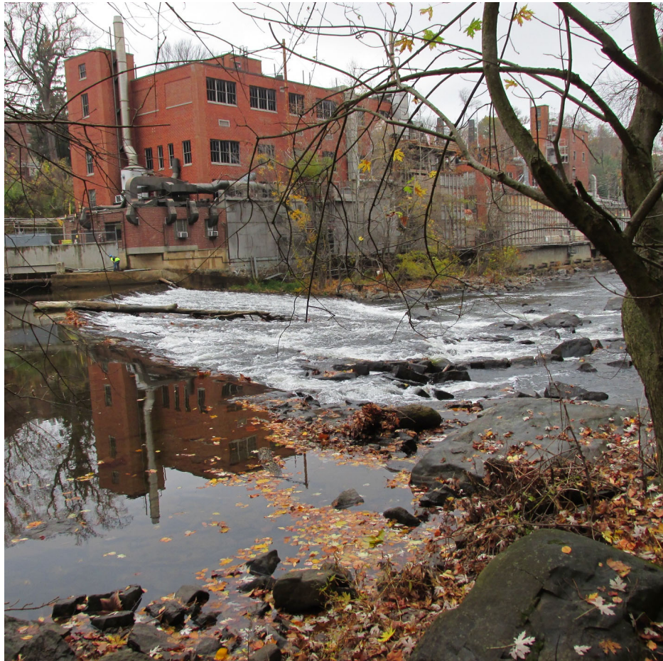
DuPont Dam 6, breached
